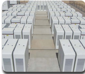
Energy storage and insulation
